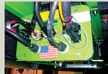
Controller and Power Inverter
